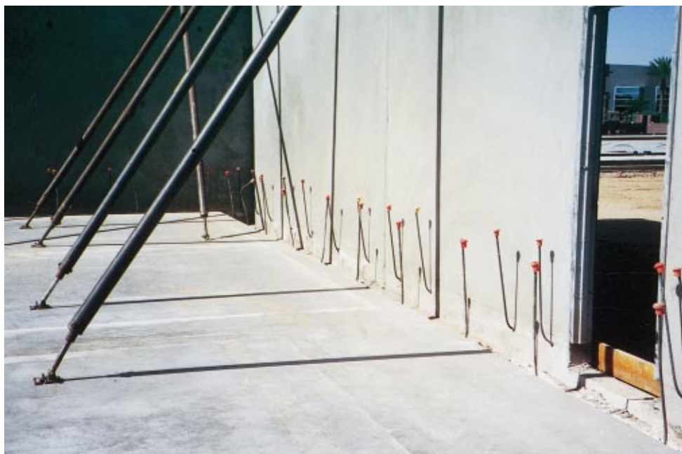
Fig. 2. (Color) Reinforcing bars extending outward from the previously placed floor slab and the tilt-up panels
