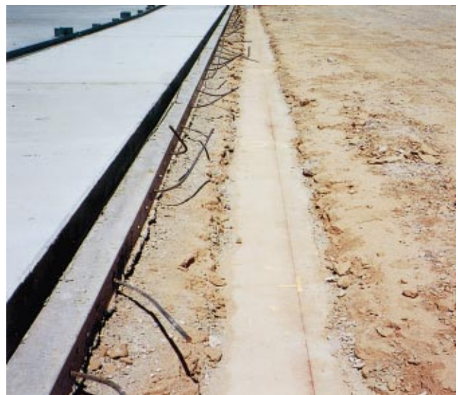
Fig. 1. (Color) Gap between the floor slab and the strip foundation
